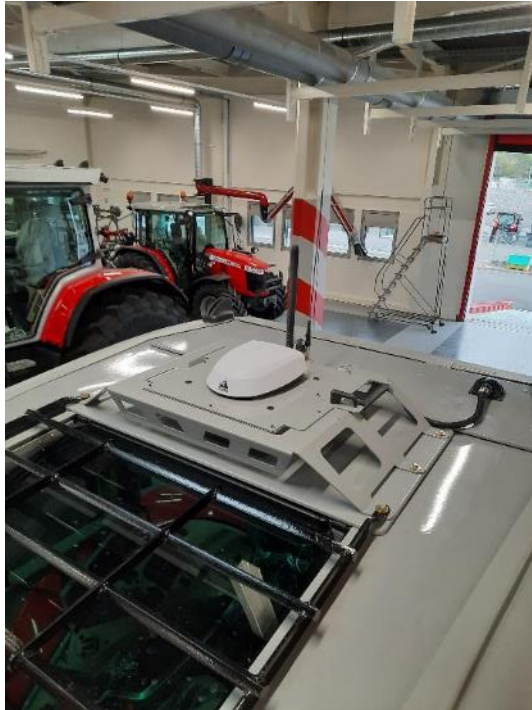
Antenna and support
